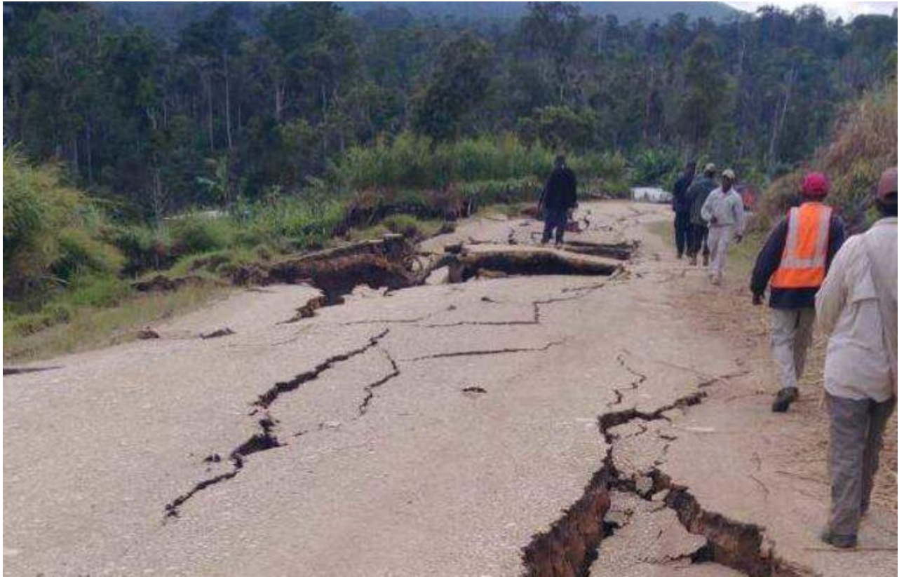
Damaged road in Komo, Hela province of Papua New Guinea, affected by the 7.5 earthquake 26 February 2018. Photo: Radio New Zealand
